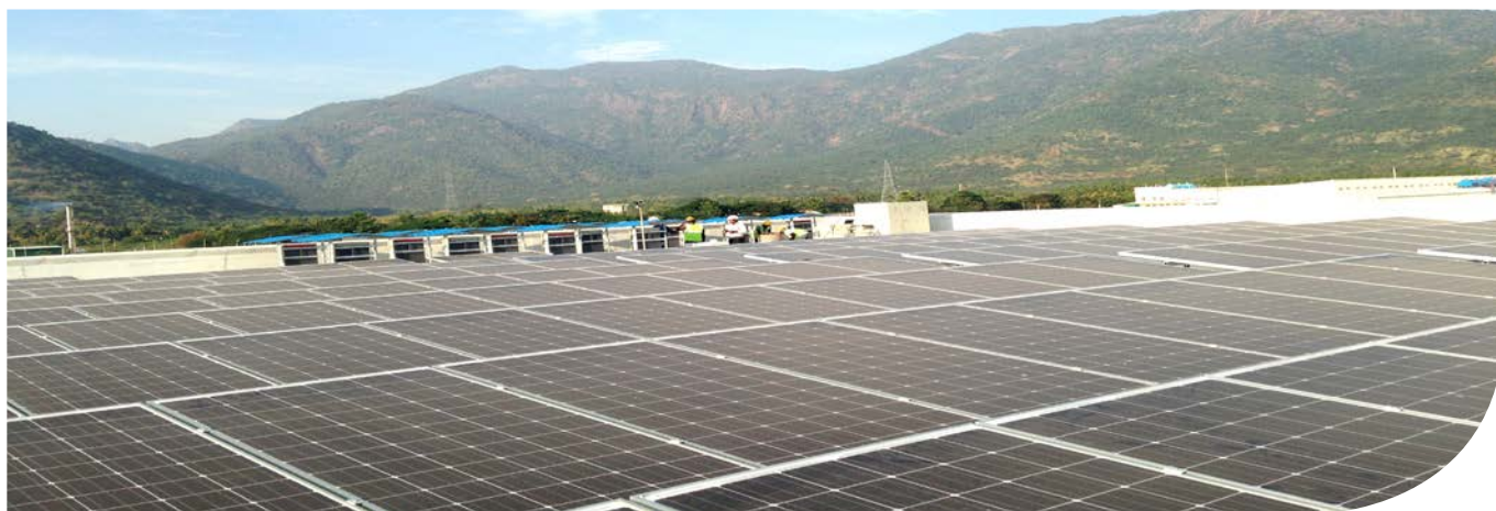
660kW PV Plant India 🇮🇳
