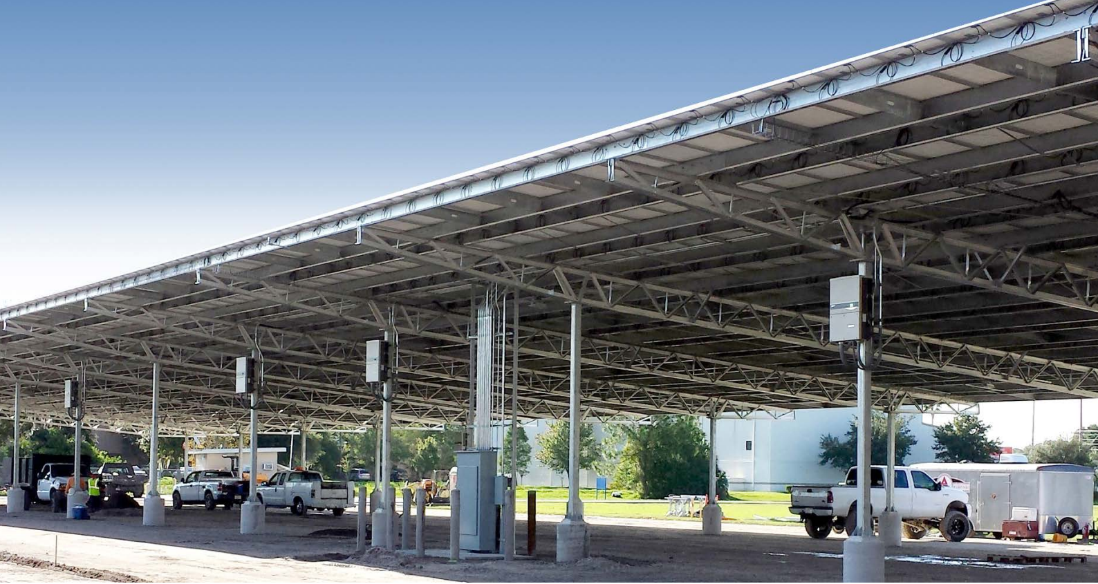
2.25 MW PV Plant USA 🇺🇸
