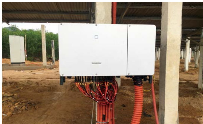
1 MW PV Plant Vietnam 🇻🇳
